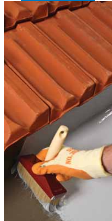
Example of a gutter waterproofed with Mapelastic Smart and coated with Elastocolor Waterproof
