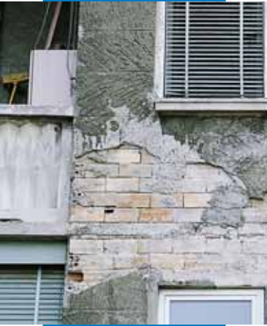
Degraded building façade in need of repair
