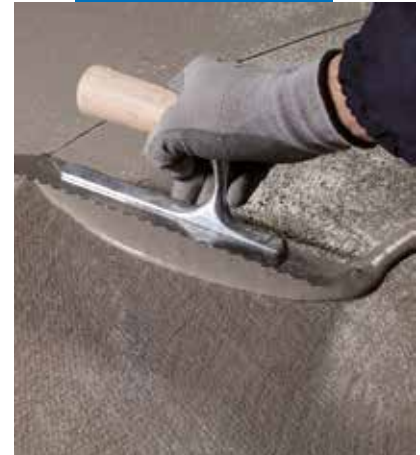
The second layer of Mapelastik Turbo over the first layer reinforced with Mapetex Sel
