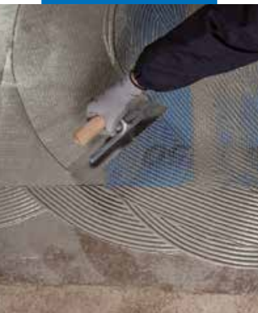
Placing Mapenet 150 on the first layer of Mapelast ic Turbo while wet
