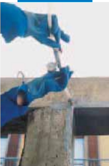
Column clad with Adesilex PG1
