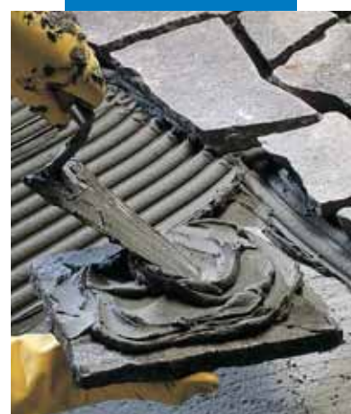
Installation of external hewn back stones with or without buttering, depending on thickness
