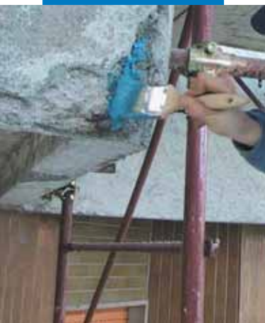
Applying Mapefer 1K with a brush on reinforcing rods of a reinforced concrete balcony
