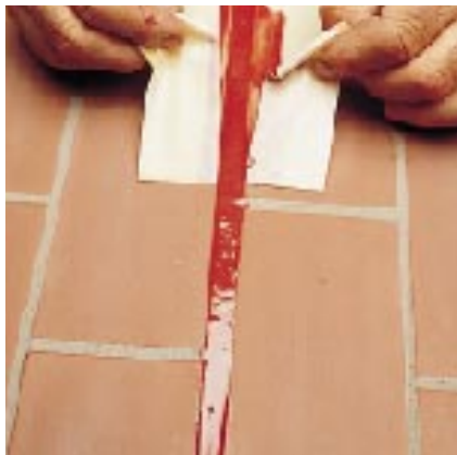
Expansion joint in red quarry tile floor sealed with MAPEFLEX PU21
