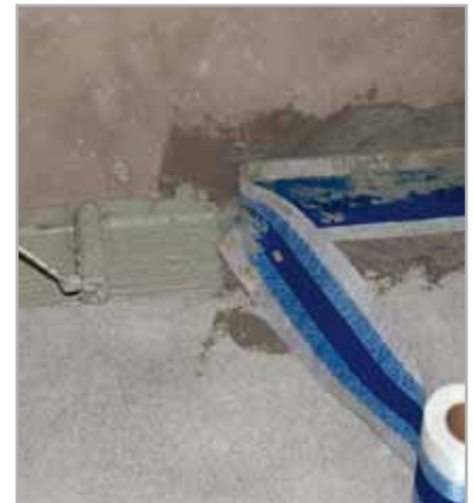
Fig 3.8 - Sealing and waterproofing fillets between a horizontal and vertical surface with MAPEBAND
